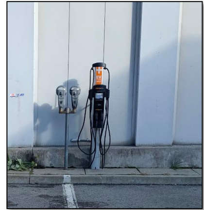
Electric car charging station, 2020
